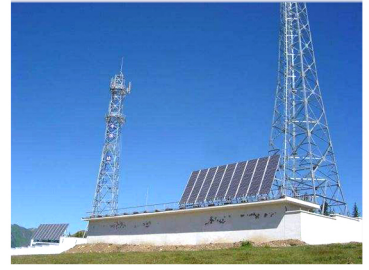
Communication base station, etc.
