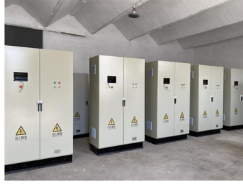
Energy storage system
