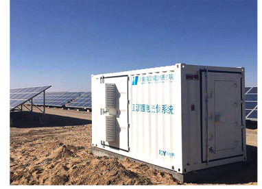
Energy storage system
