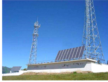
communication base station
